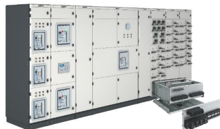
XL3 DO Distribution switchboard
